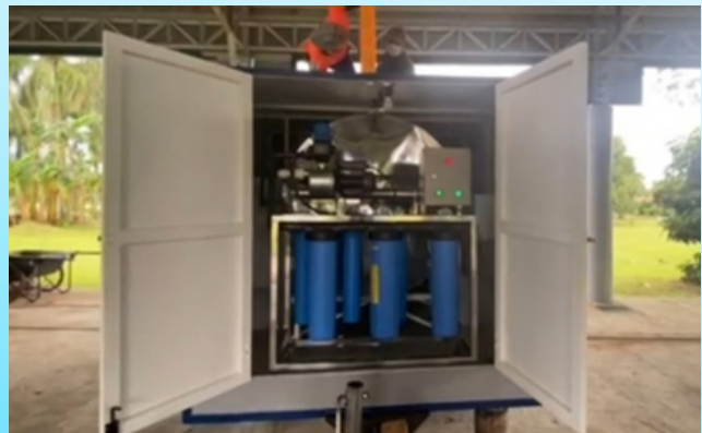
In front is the water tank and the water filtration system
