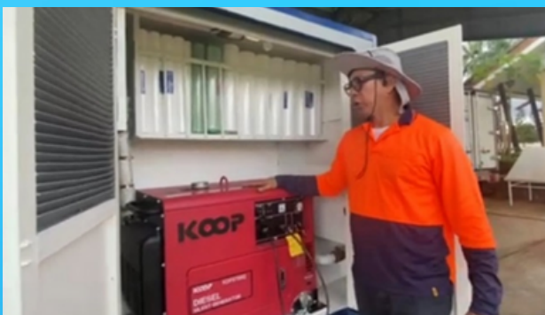
At the back is the generator and spare water filters
