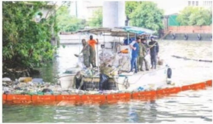
A FLAGSHIP project of the Rotary Club of Manila, the trash traps are the first of their kind to ever be installed in any of the Philippines' waterways.
