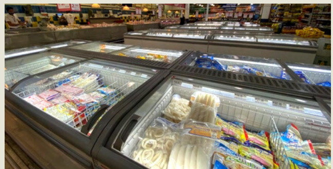
AHT island freezers and Freor showcases at Royal Duty Free Shops in Subic. It is the first R290 water loop installation in Southeast Asia and still the 'Greenest' operational store in the Philippines.
