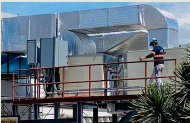
Cold Front technician in front of their installation of industrial air conditioning and ducting system
